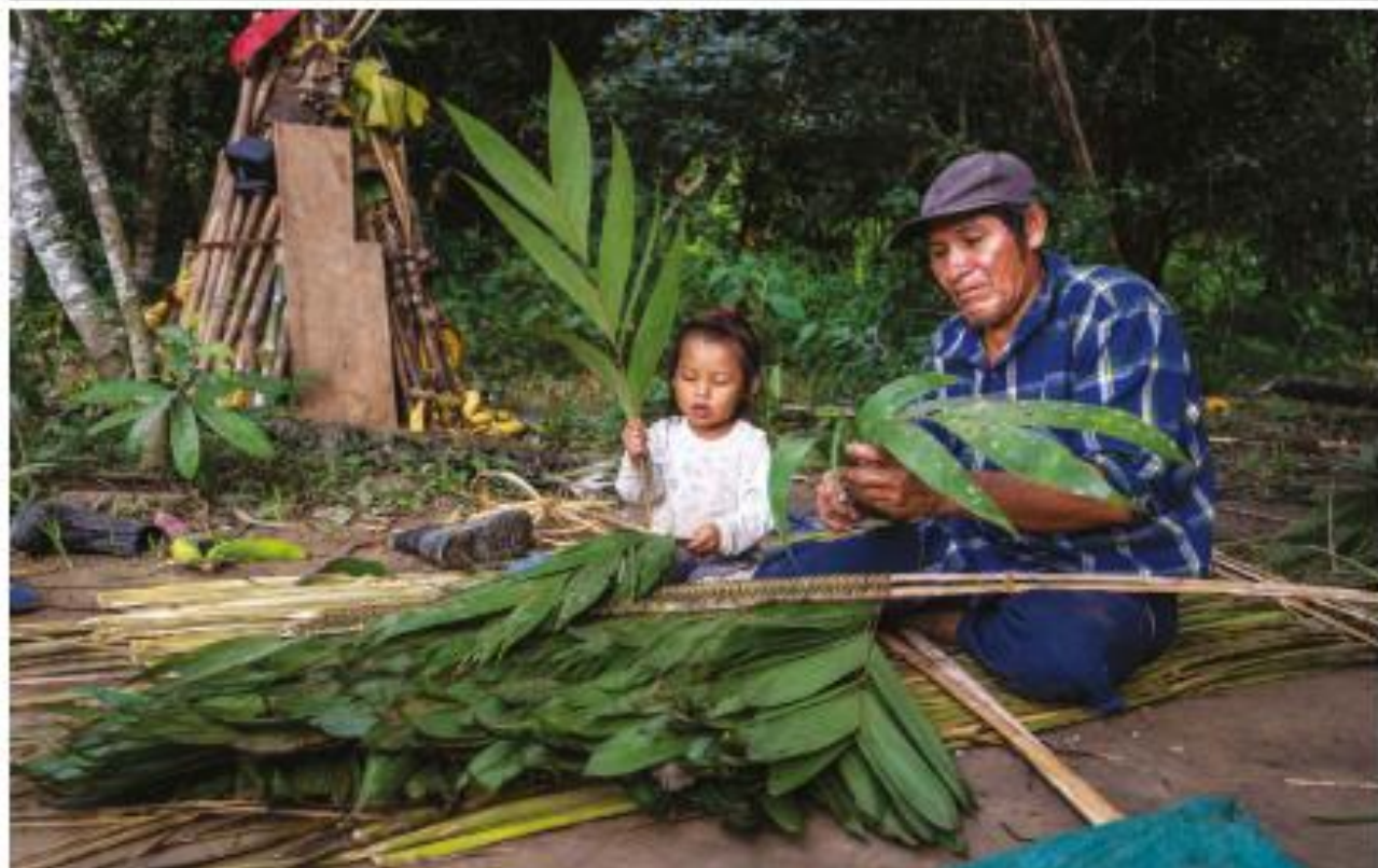
Tsimane' people in the Bolivian Amazon weave palm leaves together to thatch dwellings.
